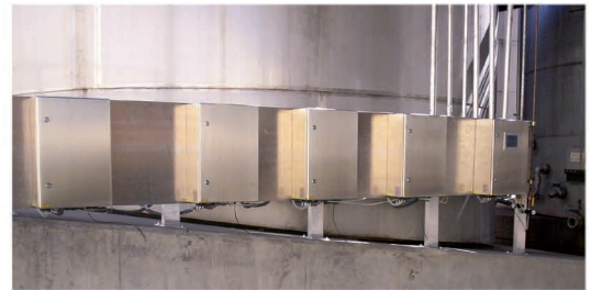
Industrial installation - 120 equipped tanks (California)
